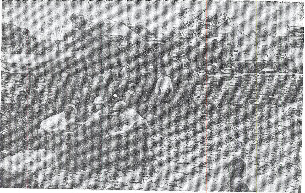
Workers salvage bricks to rebuild a Hanoi factory destroyed by bombs. Photos by Murrey Marder—The Washington Post
