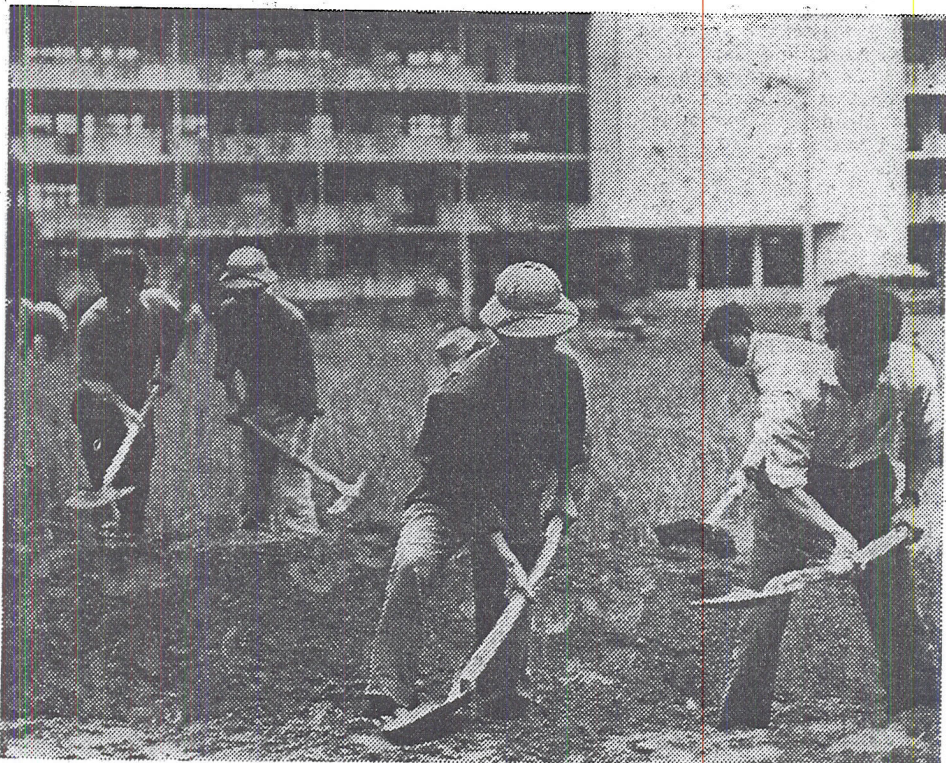
Students dig air-raid trenches on grounds of Polytechnic Institute in Hanoi after bombing raids in November. School, closed in 1966, reopened last month with 3,000 students.
