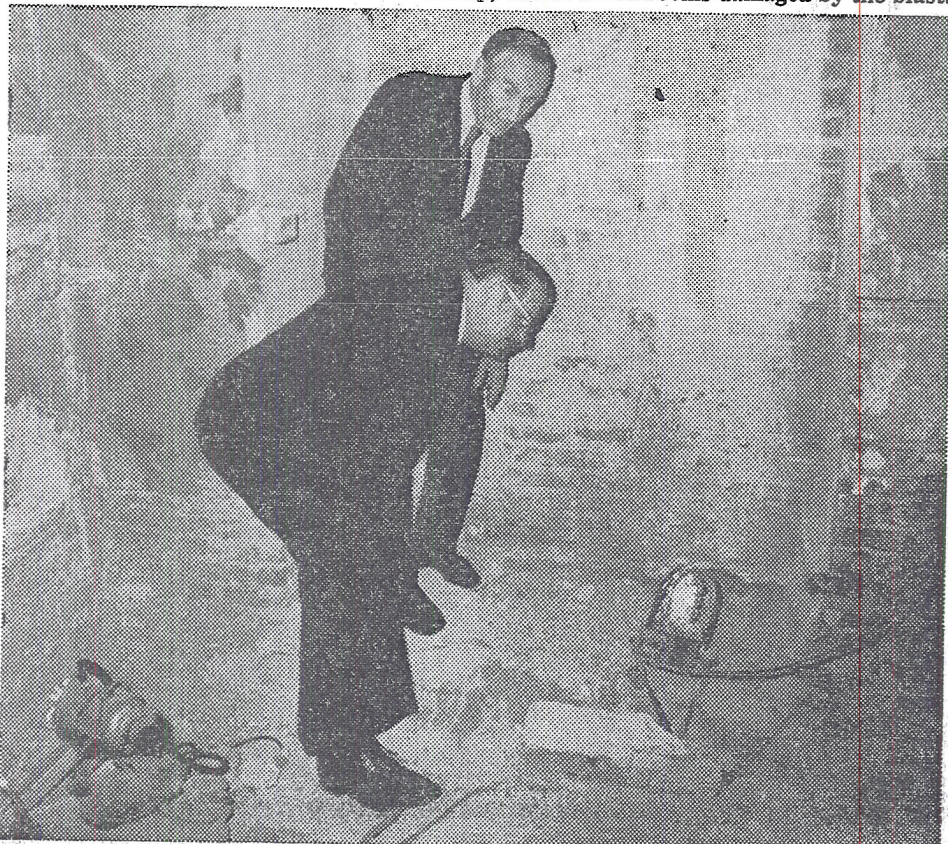
Senate leaders, Hugh Scott, Republican, foreground, and Mike Mansfield examining bomb damage in unmarked men's lavatory in basement of the Senate wing of U.S. Capitol.
