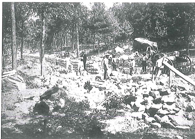
Construction of a retaining wall on Sykes Avenue, W.H. Tipton, 1897. The large rock at right center is quite visible today along Sykes Avenue.
